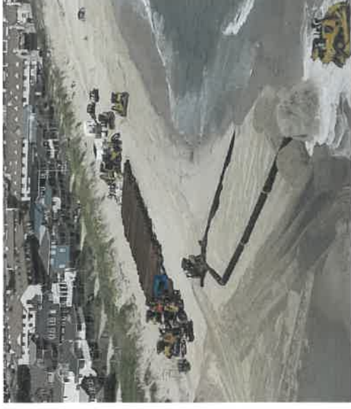
Beach nourishment was conducted for approximately 3.97 miles of shoreline from Southern Shores / Kitty Hawk town line to Kitty Hawk / Kill Devil Hills limits from August to October of 2022 at a cost of $9,600,000.
