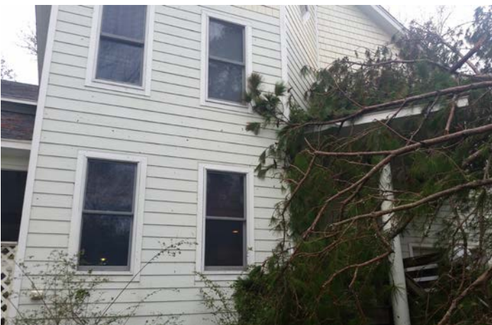
Fallen tree from Hurricane Matthew in October 2016
